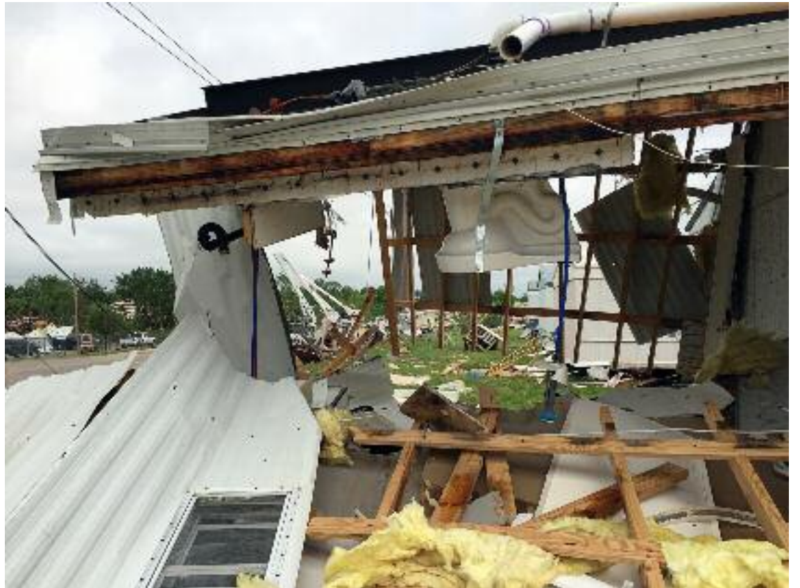
A toilet seemingly hangs from the ceiling in this trailer that was completely picked up by powerful winds, flipped upside down and smashed into another trailer nearby. Photo Tom Welte
