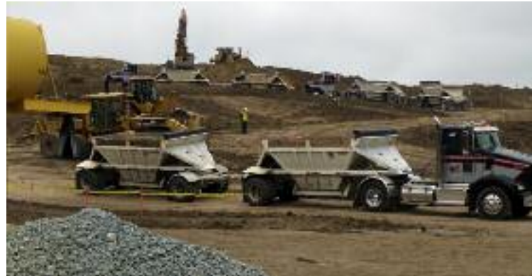
Trucks line up to remove excavated dirt from the Camino Ricardo subdivision. Photo Sophie Braccini
