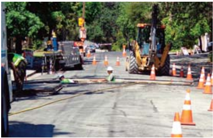
Brook Street is closed near Moraga Road for EBMUD, where workers are replacing over 500 feet of pipe that was installed in 1933. Photo Cathy Tyson
