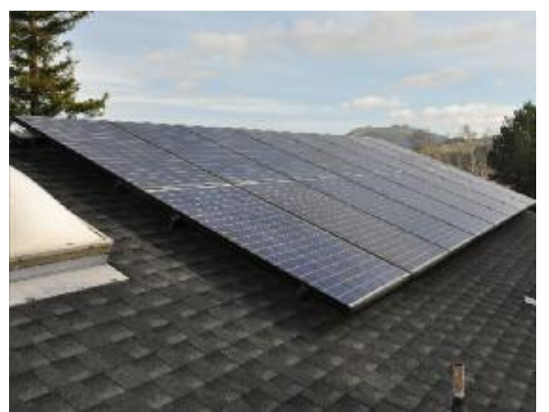
Solar panels on rooftops
