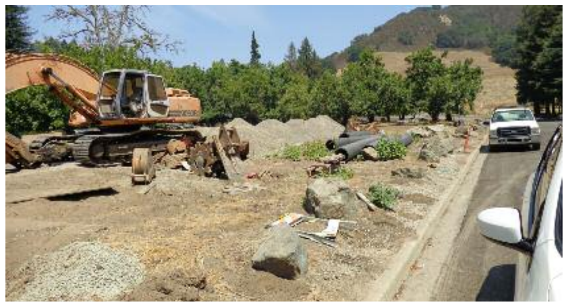
Heavy equipment and pipes that are part of storm drain upgrades on newly formed subdivision on Franklin Lane. Photo C. Tyson
