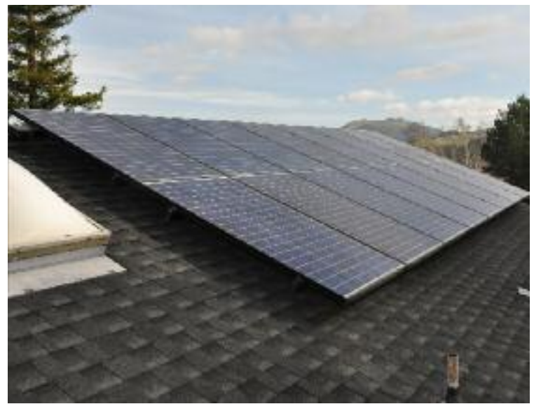
Solar panels on rooftops
