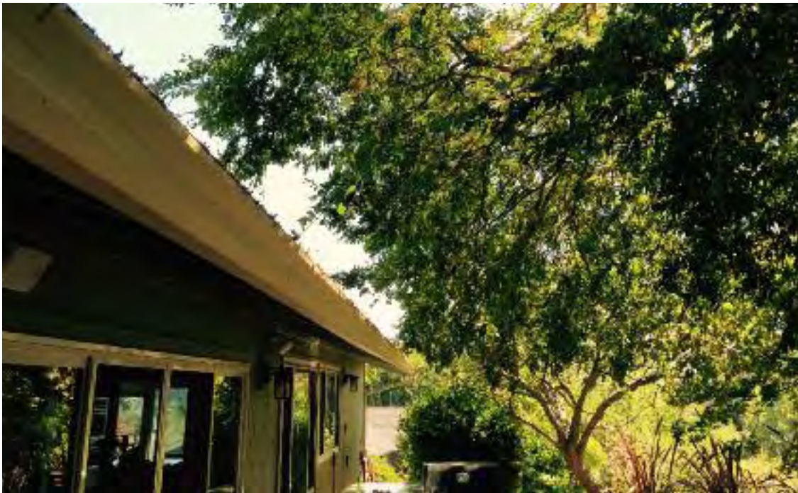
Tree limbs hanging over a roof is a no-no.
