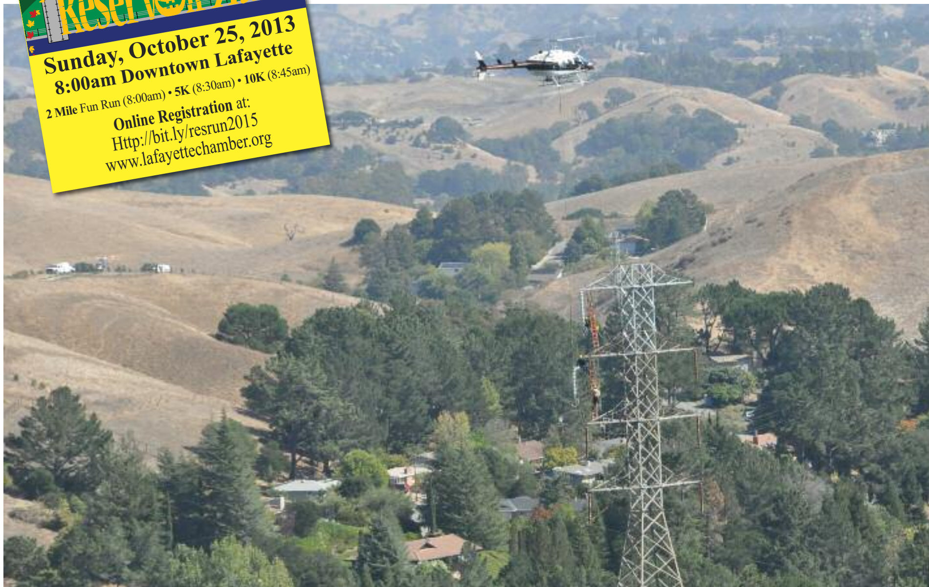
Specially trained linemen stand atop PG&E's lattice steel structures after being lifted by the helicopter hovering above.
