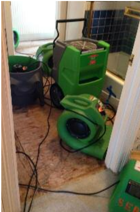
Water damage was extensive at Cynthia Brian's home. Photos courtesy Cynthia Brian
