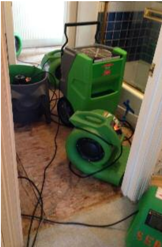
Water damage was extensive at Cynthia Brian's home. Photos courtesy Cynthia Brian
