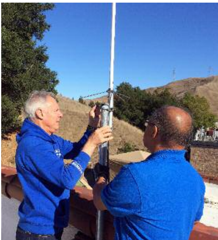
LARIG volunteers Dan Spisak, left, and Al Archangel install a multi-purpose antenna at 335 Rheem Blvd. Photo Cathy Dausman
