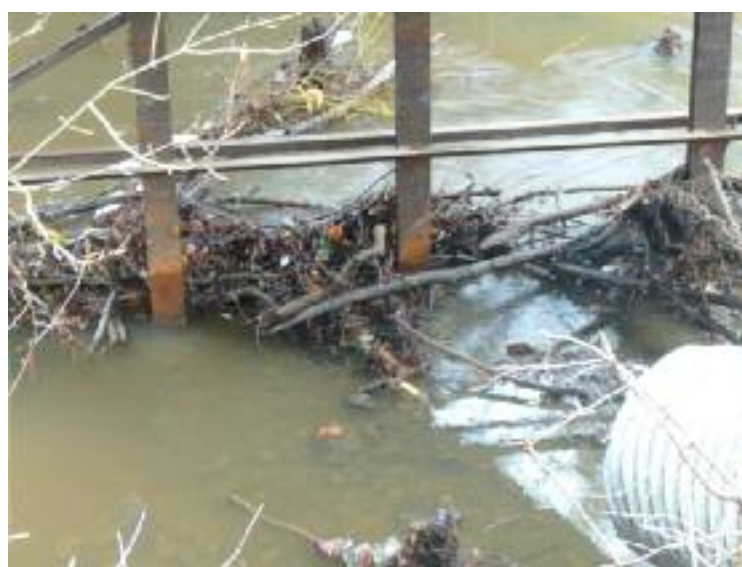
More debris under the Canyon bridge
