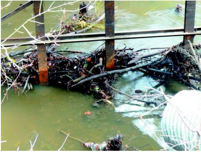
More debris under the Canyon bridge
