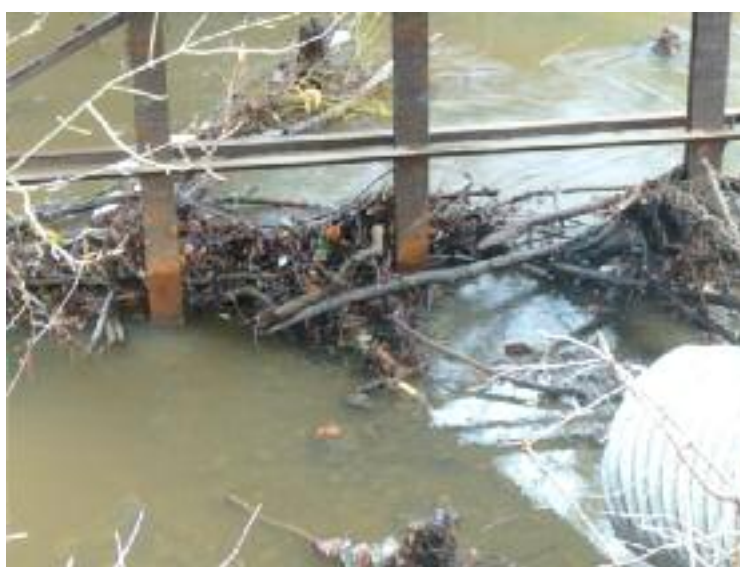
More debris under the Canyon bridge
