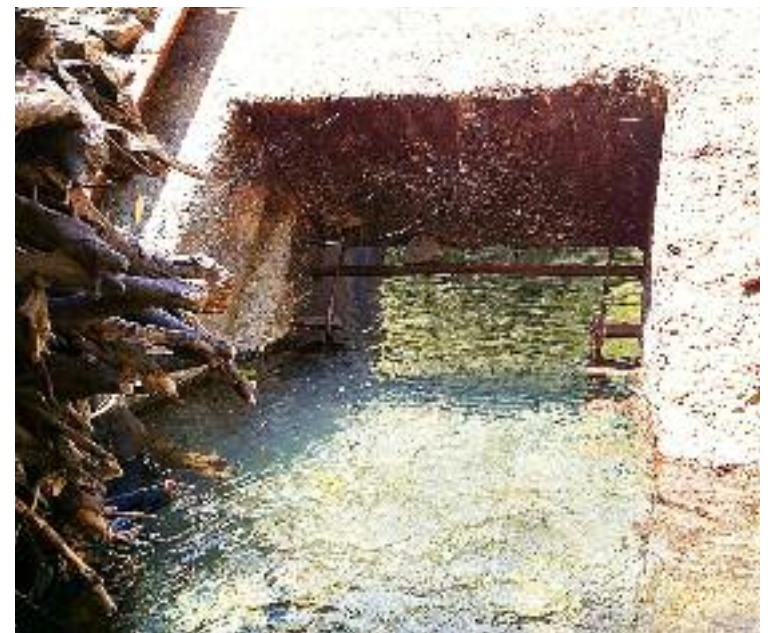
The opening in the drop structure on upper San Pablo Creek unexpectedly blew out last fall, which would have allowed fish to migrate up into its native waters. The opening is clogged again.
