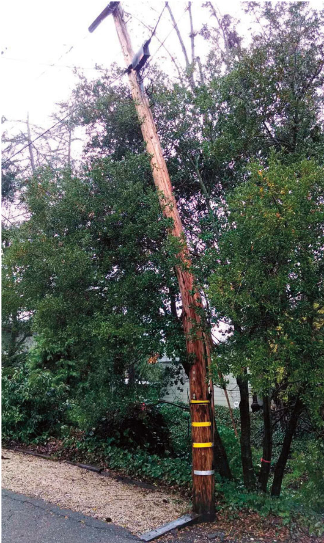
A damaged power pole after recent storms Photo Dana Farkas
