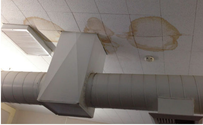
Ceiling water damage at a Lafayette school. Photo provided
