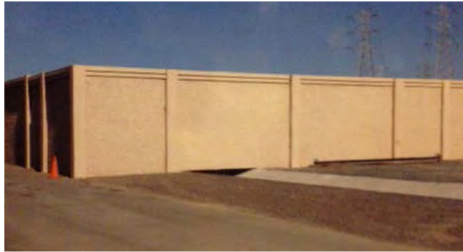
This image of a masonry security wall was presented at the meeting. Image provided
