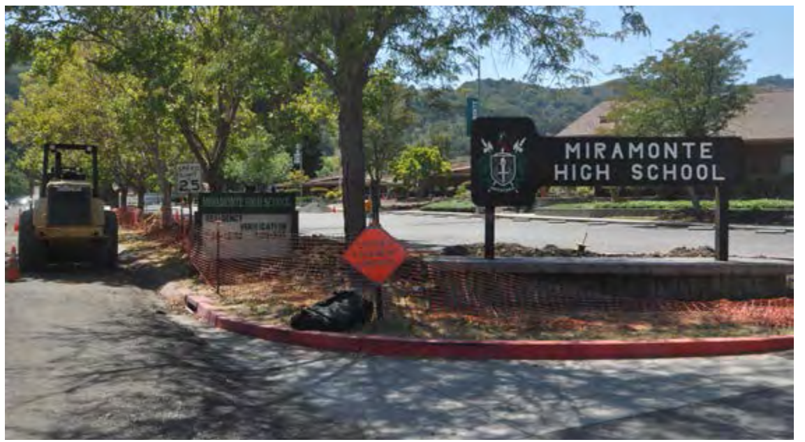
The road, sidewalk and parking lot at Miramonte High School are still under construction. Photo Andy Scheck
