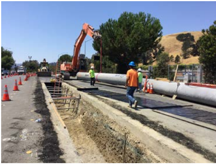
A 30-inch pipe is currently being installed on Mt. Diablo Boulevard. Photos courtesy EBMUD
