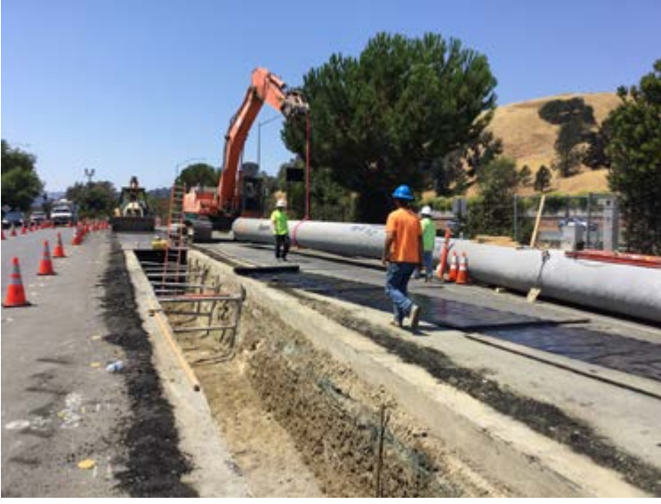
A 30-inch pipe is currently being installed on Mt. Diablo Boulevard. Photos courtesy EBMUD
