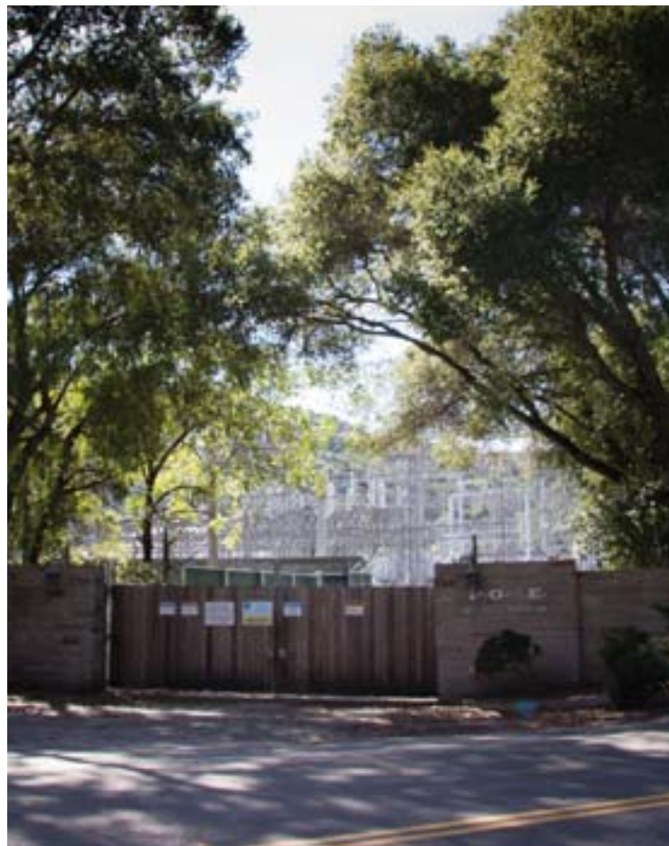
The Lost Valley PG&E substation.
