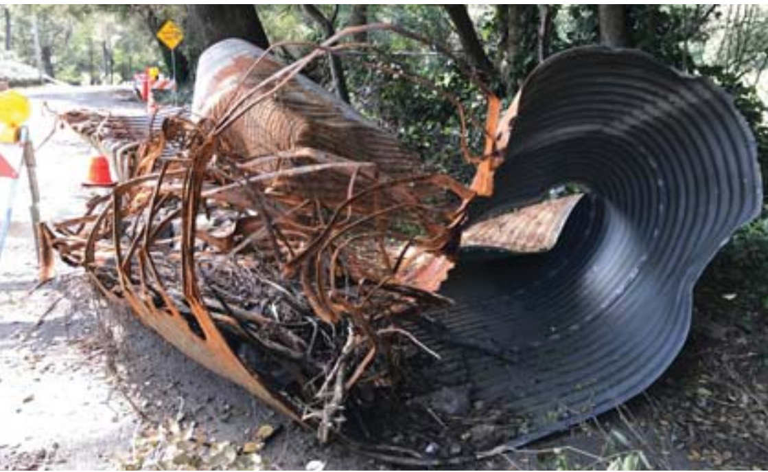
This damaged pipe underscores the severity of the sinkhole.
