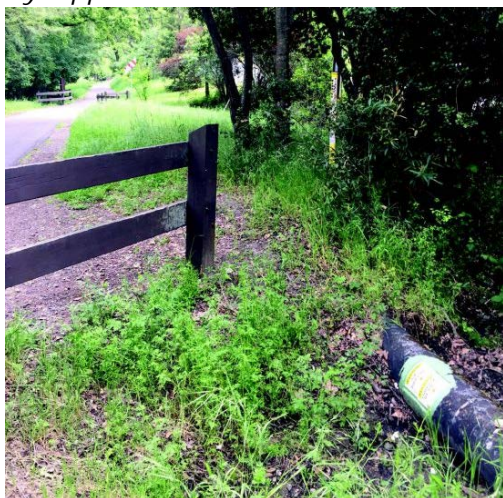
An exposed gas line along the Lafayette-Moraga Trail. Photo P. Fisher
