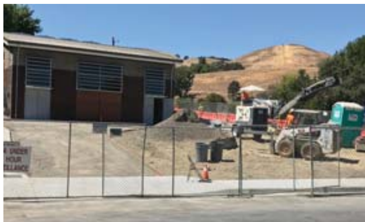
EBMUD's new Diablo Vista pumping plant set to be operational by early 2018. Photo Pippa Fisher
