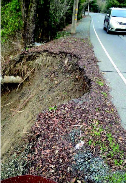
St. Mary's Road at the point of slide - exposed pipe visible. Photo provided
