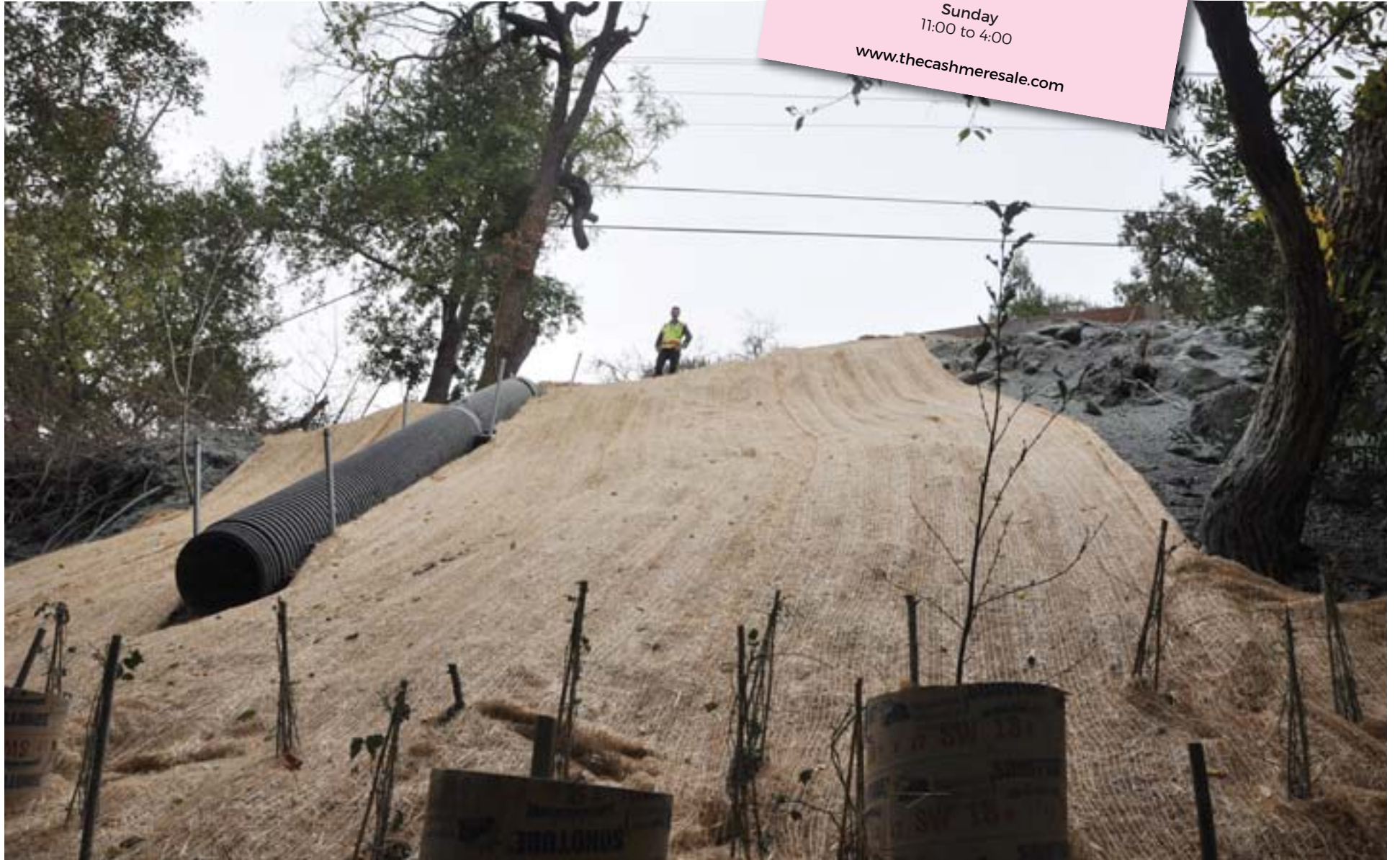
Mike Moran looks down at the 40-foot slide area. Left: the new drainage pipe sits behind newly planted trees along the creek bed.
