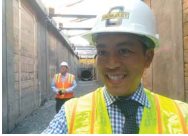
Moraga Public Works Director Edric Kwan with Project Manager Senior Civil Engineer Shawn Knapp in the trench as the culvert is repaired.
