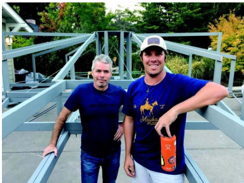
Working on a classic: Powell's neighbor Michael Ferrif and friend Bob Christopher inside the framework.
