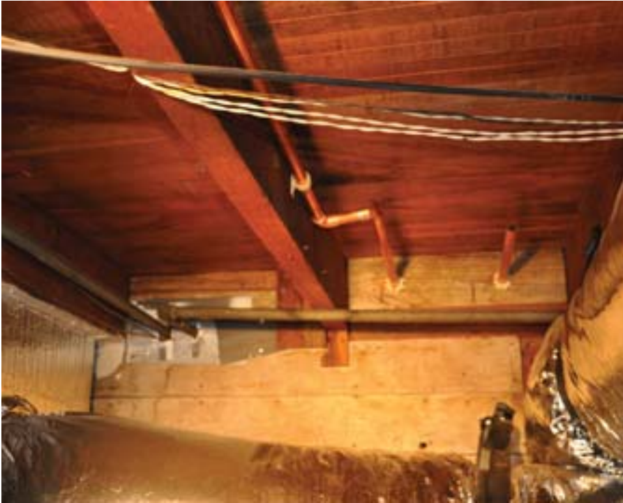
New copper piping on top and old pipes below.
