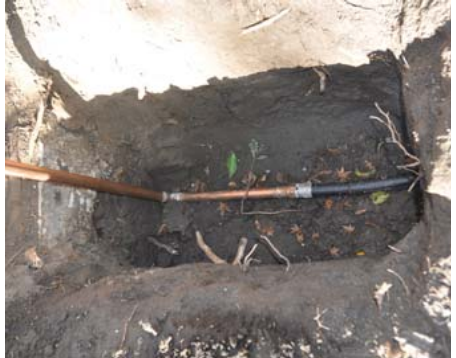
The new copper pipe is connected to the water main outside the house.
