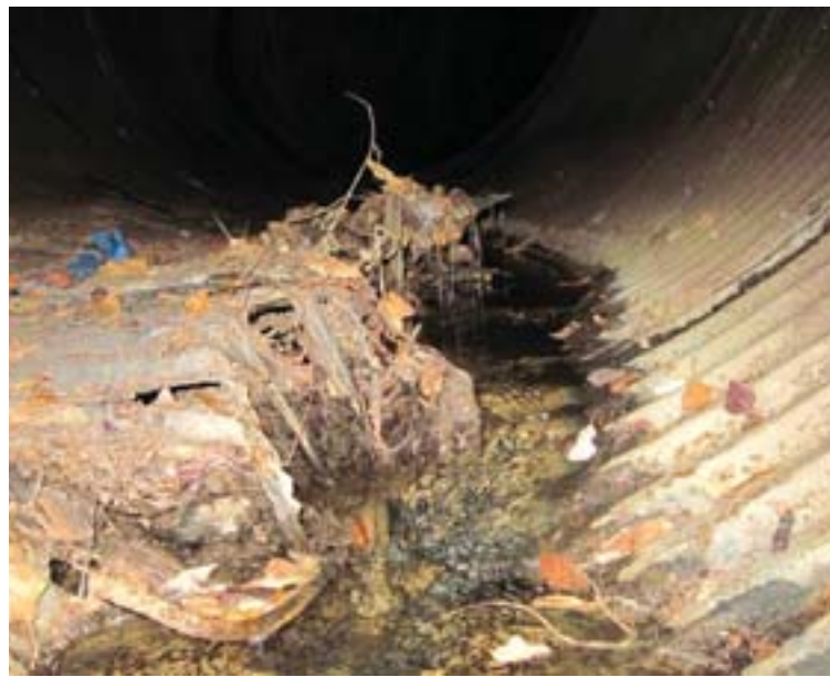
A broken pipe eight feet upstream at Rheem Boulevard and Center Street Photo provided
