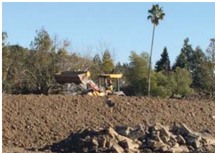
KB Homes grades the future site for the Moraga Center Homes. Photo Sophie Braccini
