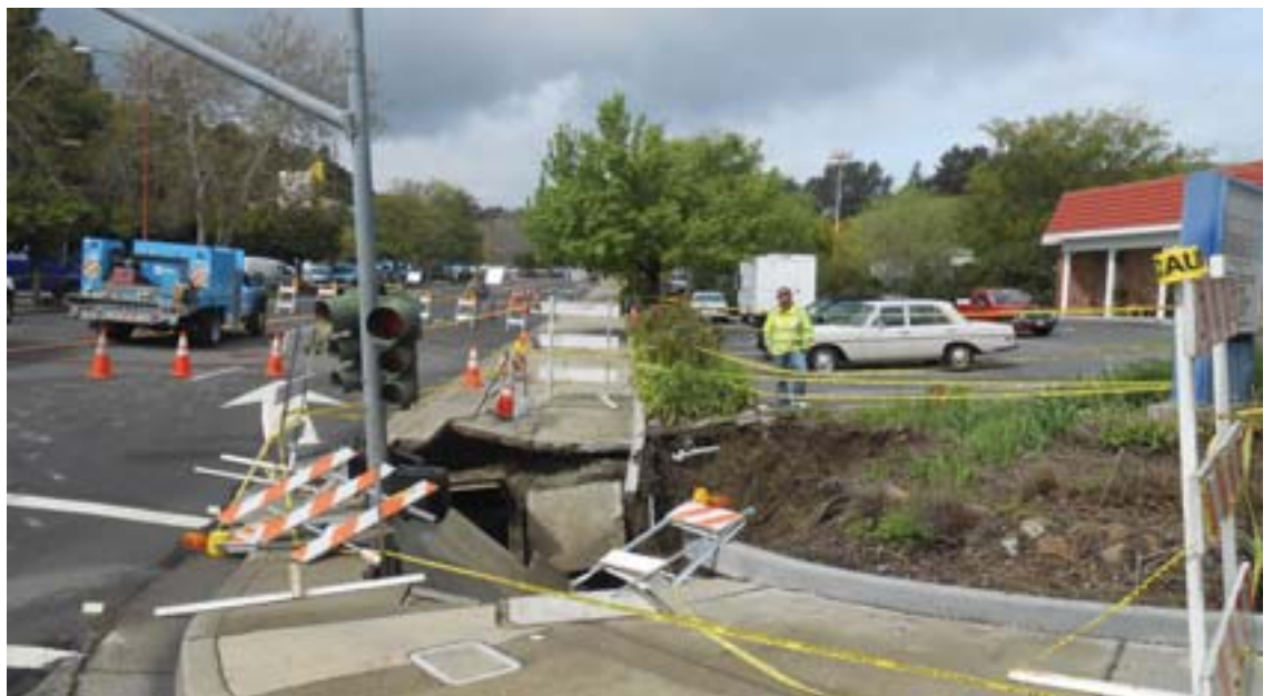
This sinkhole developed in March 2016 Photo provided
