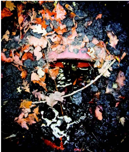
A clogged drainage pipe Photo Sora O'Doherty
