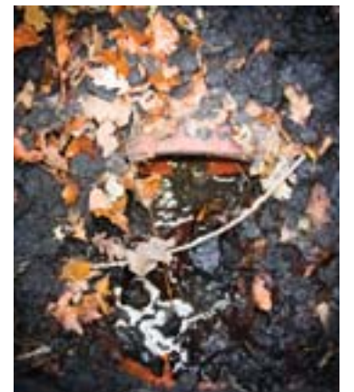
A clogged drainage pipe
