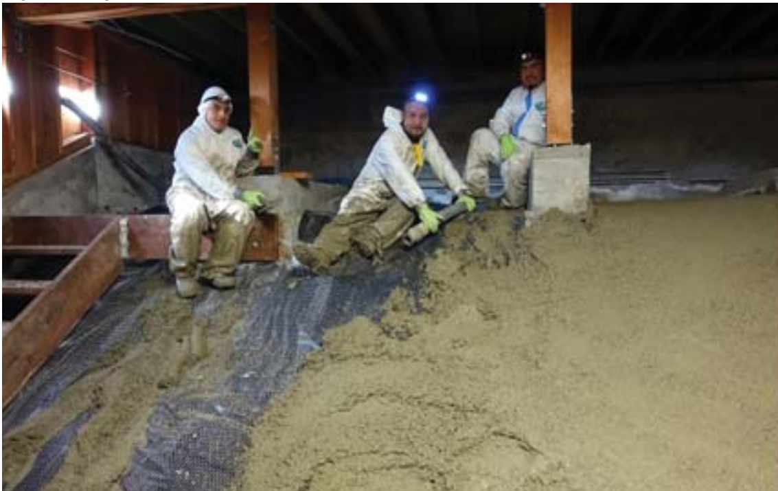
Pouring concrete over crawl space, especially on an underground incline, is hot and dirty work.
