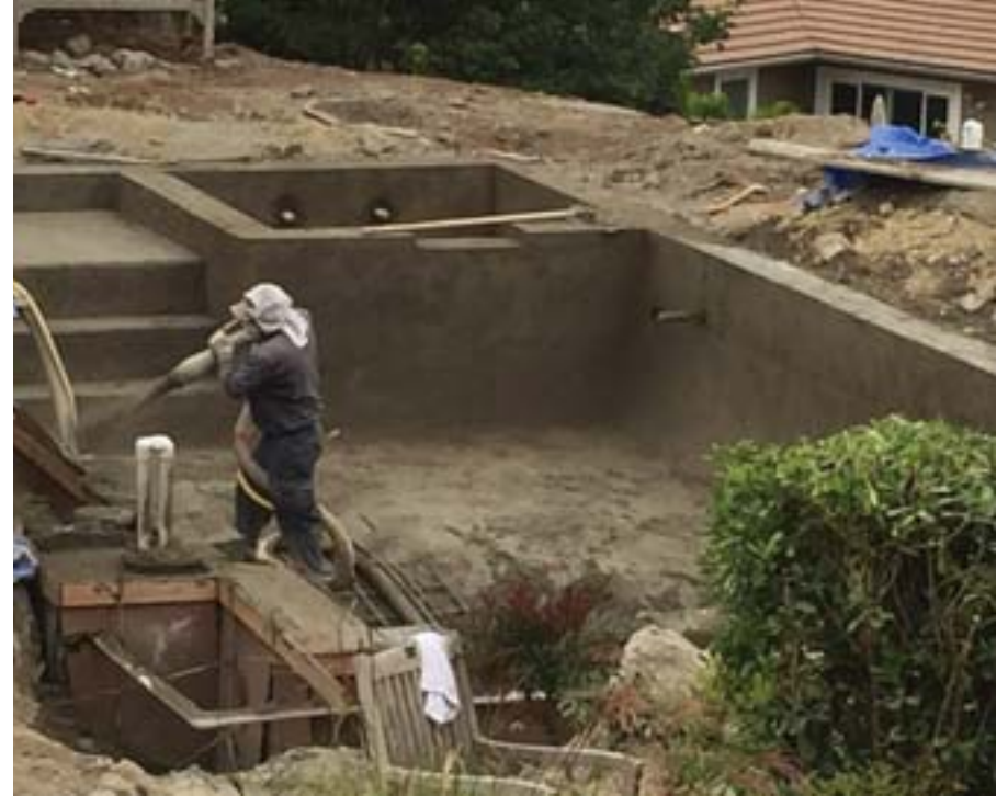
Gunite is sprayed over steel rebar forming the pool shape. Oversized first step is called a sun shelf.
