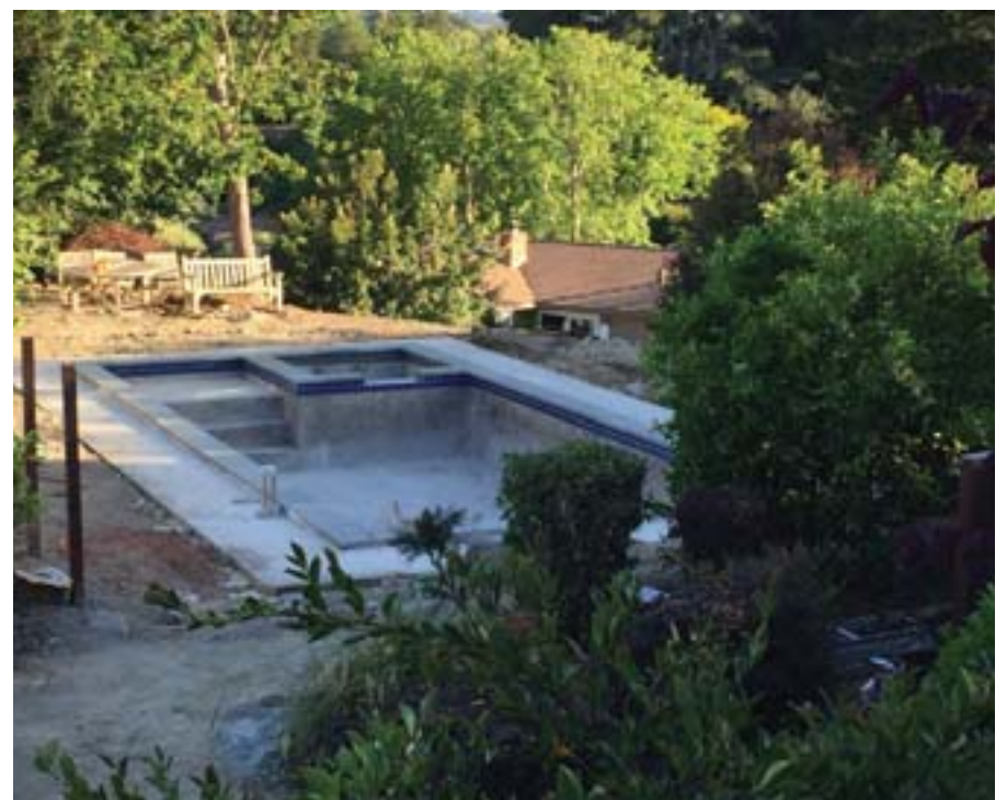
Decorative tile installed; Pennsylvania blue stone used as coping stone is mortared to the top of pool.
