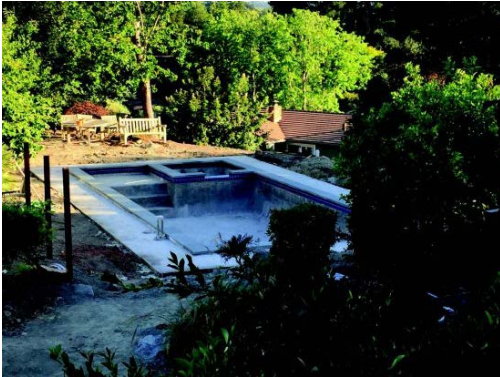
Decorative tile installed; Pennsylvania blue stone used as coping stone is mortared to the top of pool.
