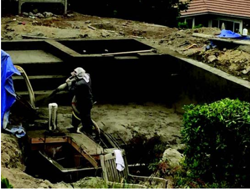
Gunite is sprayed over steel rebar forming the pool shape. Oversized first step is called a sun shelf.
