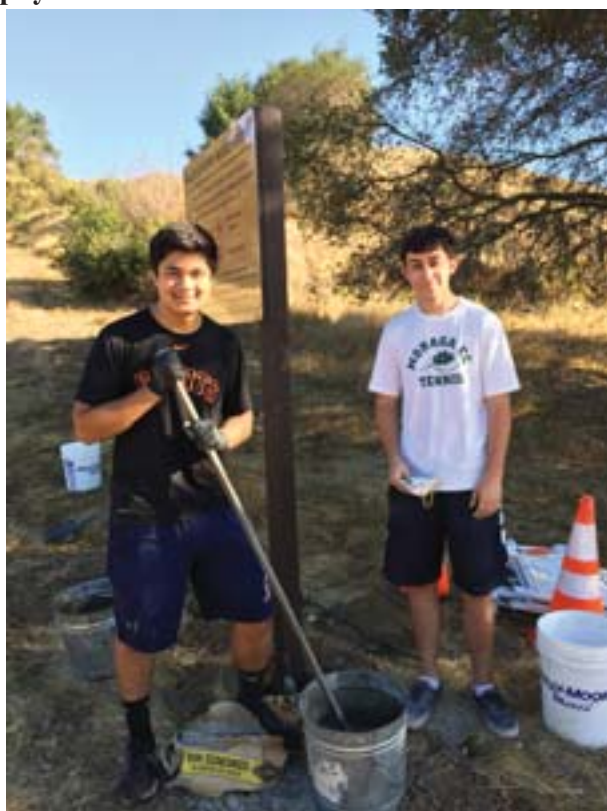
Campolindo senior Alex Mangoba (left) is assisted by fellow Boy Scout Andy Babson in installing a new sign along the Lafayette Reservoir Rim Trail. Photo Linda Murphy
