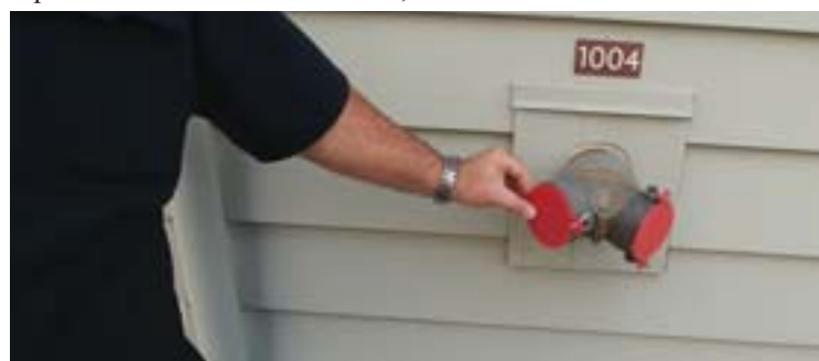
Aubert tests the fire department connection.
