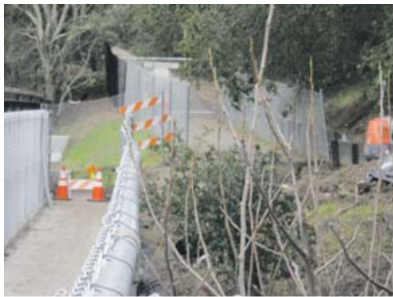
Canyon Bridge pedestrian access closed
