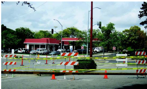
Cordoned off area of sinkhole Photos Vera Kochan
