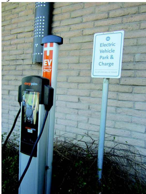
Electric Vehicle charging ports in use at one of Lafayette's locations Photo Vera Kochan
