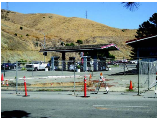
Rheem sinkhole still awaits repairs. Photo Vera Kochan
