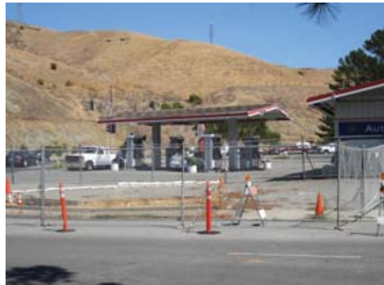
Rheem sinkhole still awaits repairs.
