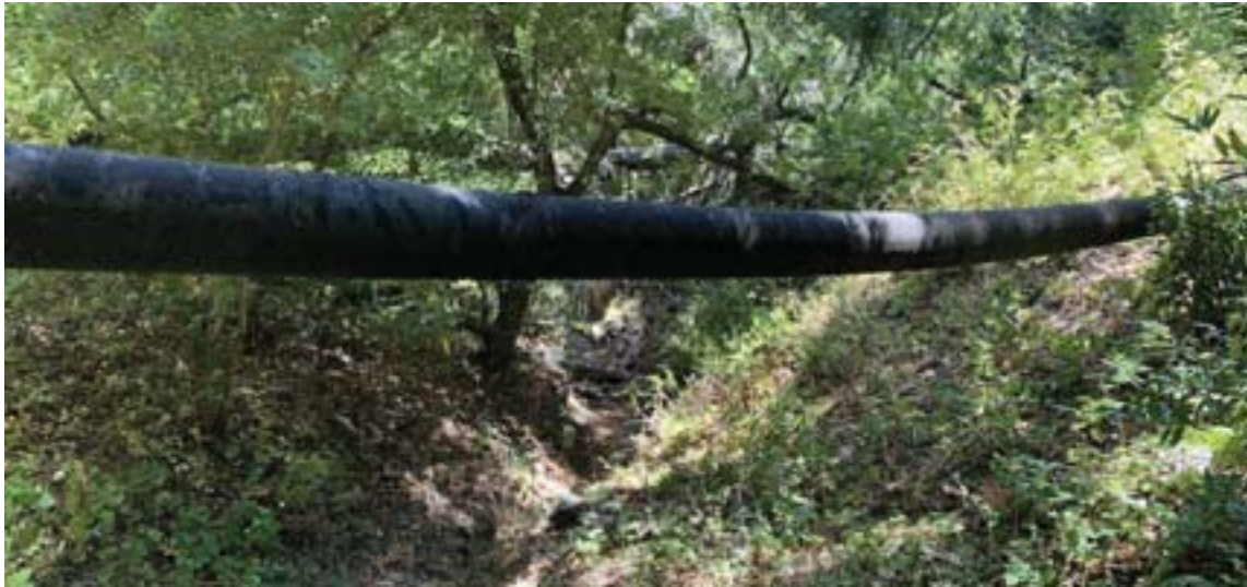
The exposed, high-pressure PG&E pipeline near the Springhill neighborhood is unsupported at each end and sags mid-span.
