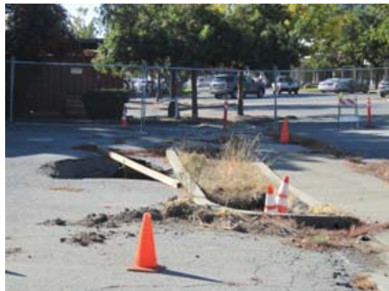
Rheem sinkhole gets larger
