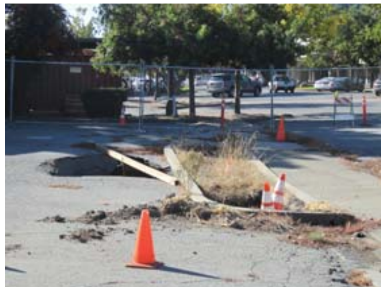
Rheem sinkhole gets larger
