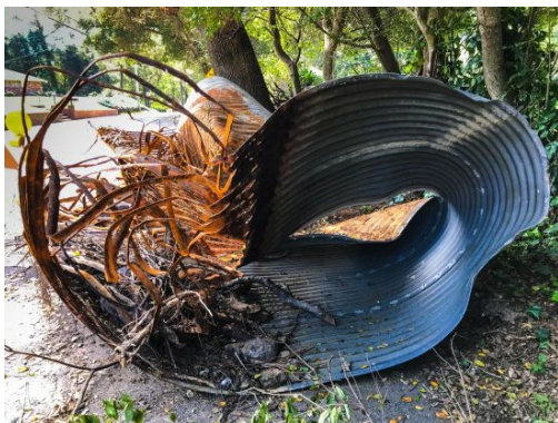
Failed metal culvert that was replaced with concrete culvert under Miner Road in 2017. Photo Sora O'Doherty
