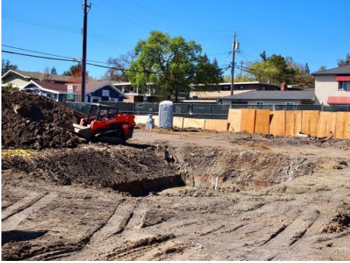
On Brown Street crews have started grading. Once site work is complete they will start the vertical construction. Photo Pippa Fisher
