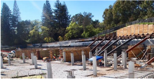
Work has started on the Lennar project in earnest now. Photo Pippa Fisher
