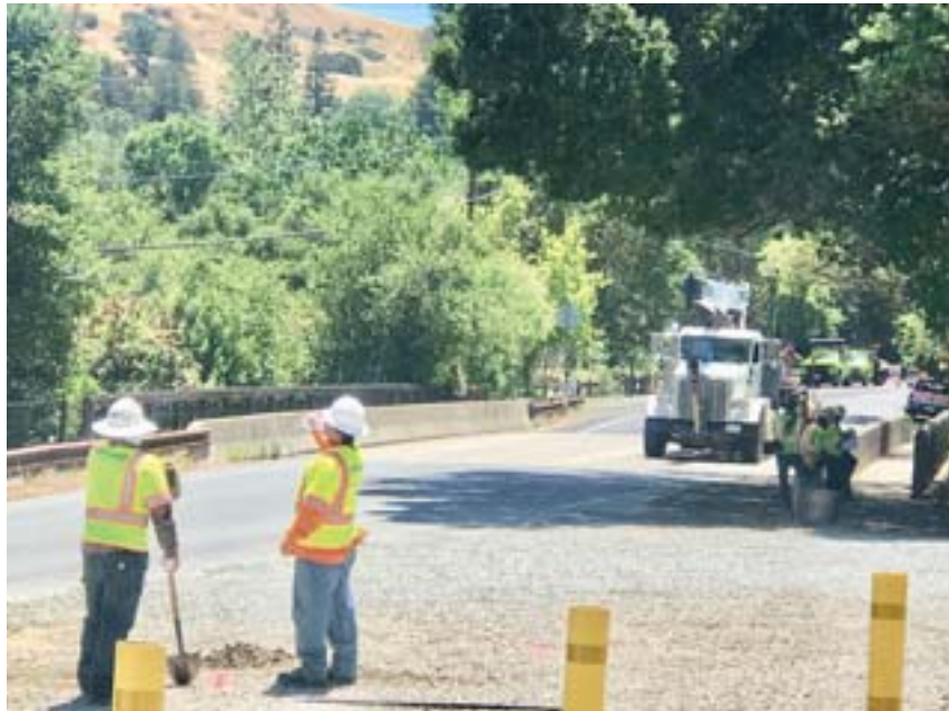
PG&E work began June 1, with tree removal planned to start the week of June 15.
