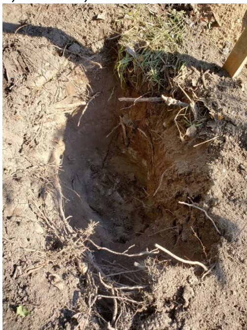
Large postholes are needed for sturdy fence post installation. Photos Jim Hurley
