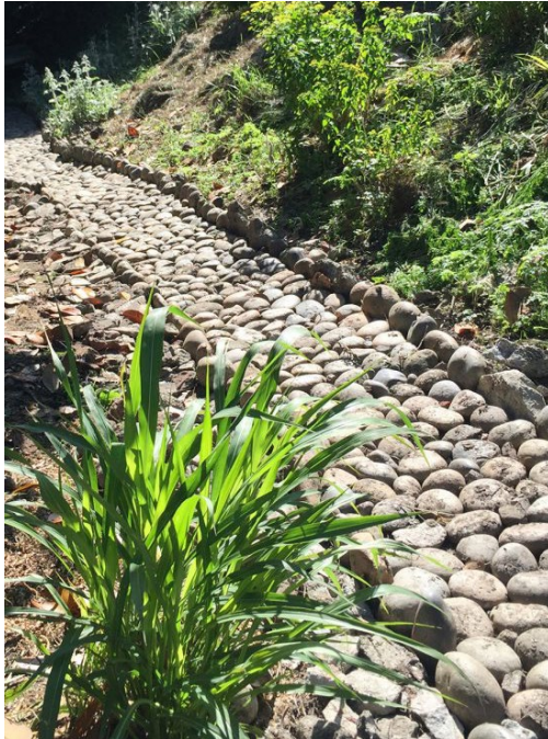
A river rock canal provides some protection near structures. Photo Cynthia Brian
