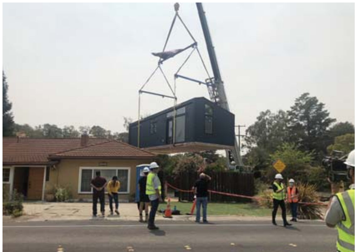
A crane lifts the ADU over the side fence into the backyard.
