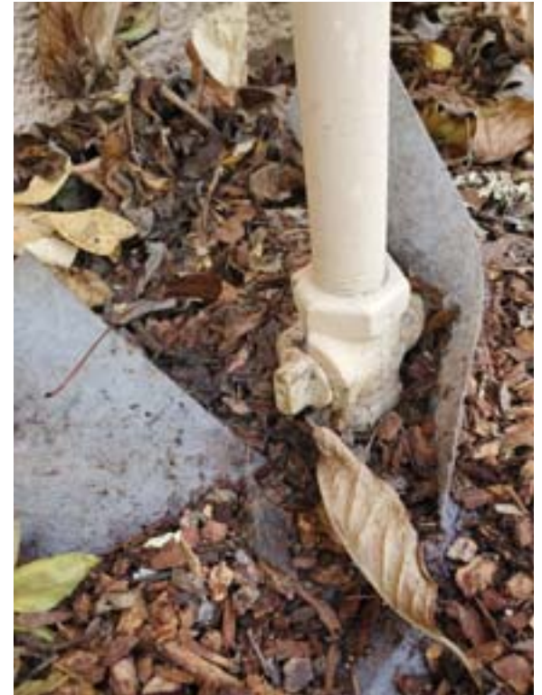
Gas shutoff valves
