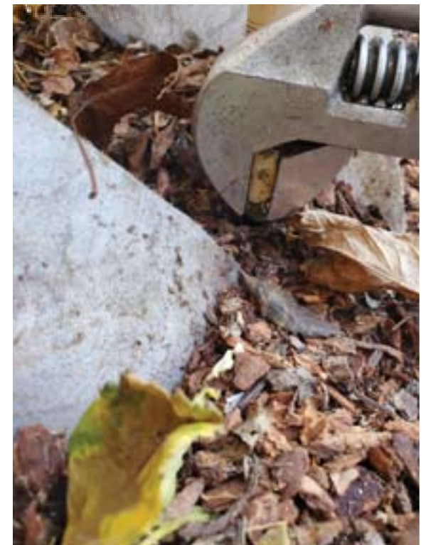
Gas shutoff valves can be closed with a wrench
