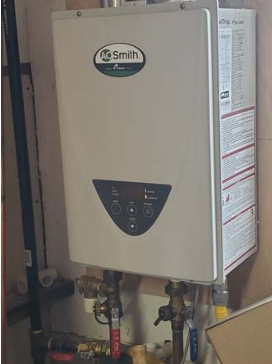
On demand water heater
